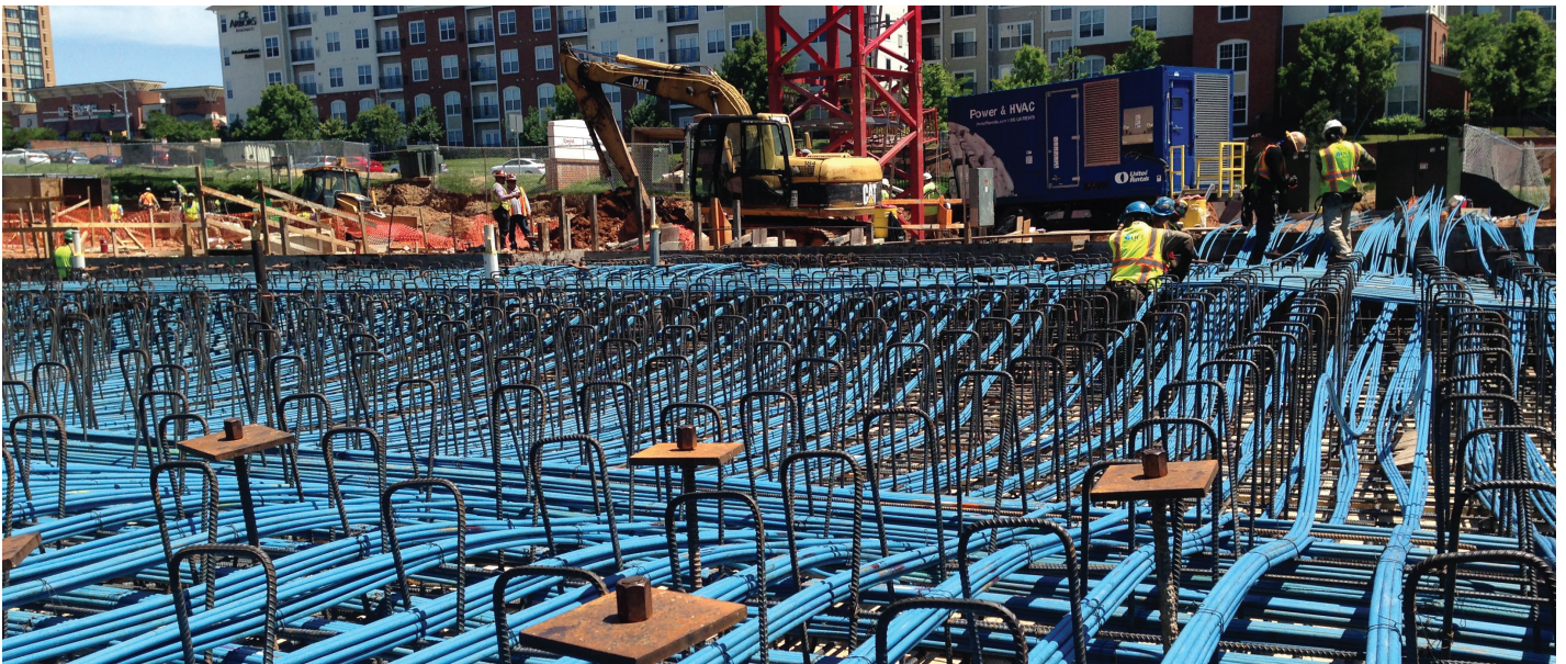
Fig. 4—Transfer mat foundation spanning over SWM tanks. This photo shows post-tensioning cables that are profiled with high points over the piles and low points at midspan. The underground tanks are in the middle section of the mat.
