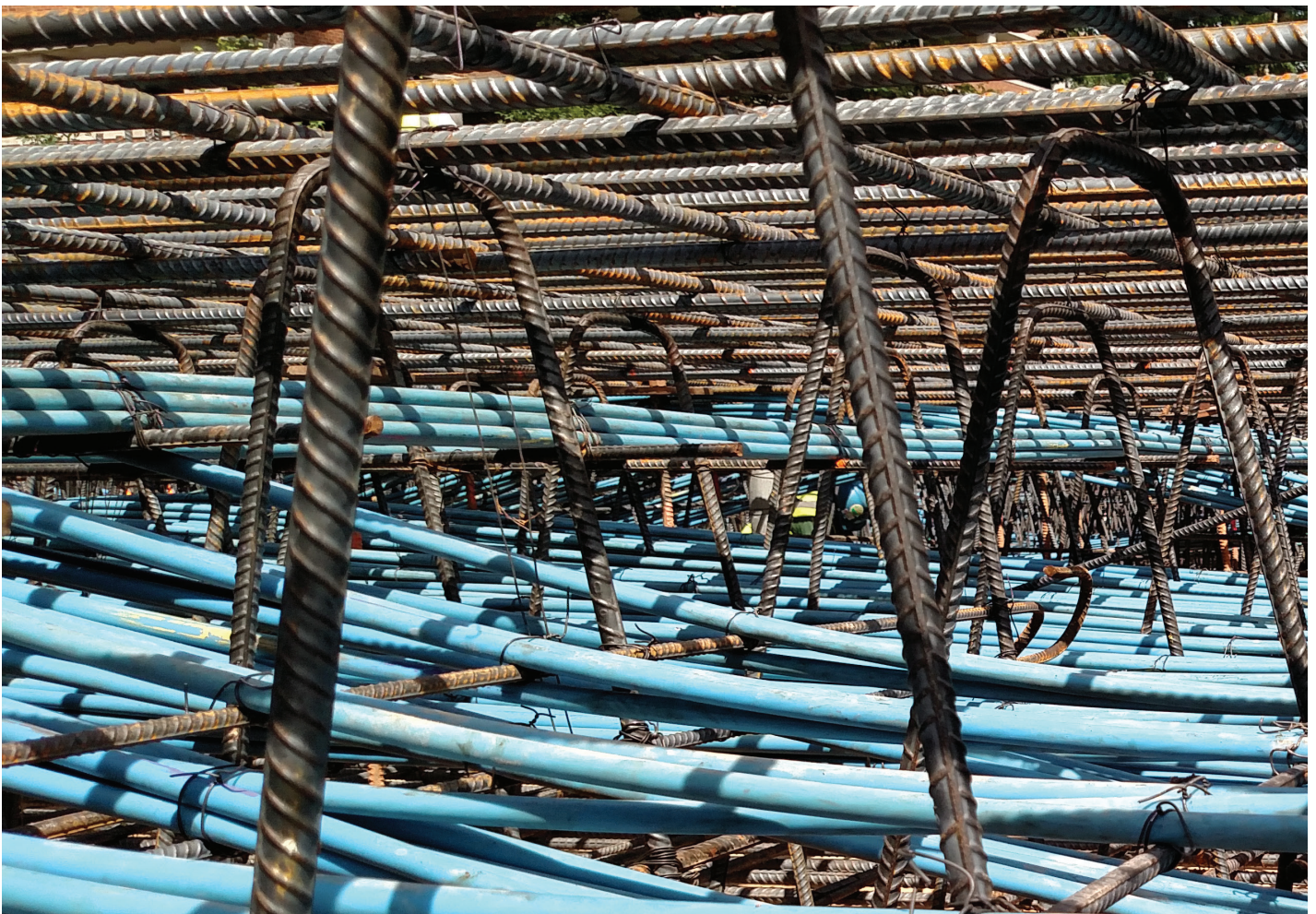
Fig. 5—View of reinforcement between top and bottom mat of steel in transfer mat.
