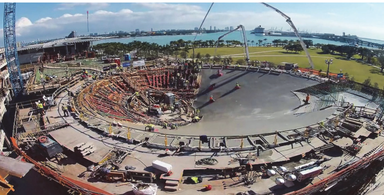
b. Concrete placement using single and double-sided wall forms. Fig. 7—Tank under construction.
